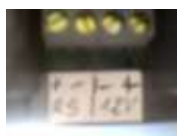
Fig. 2.1. View of the room panel back side where conductors are connected according to the description found in section 2.1.
